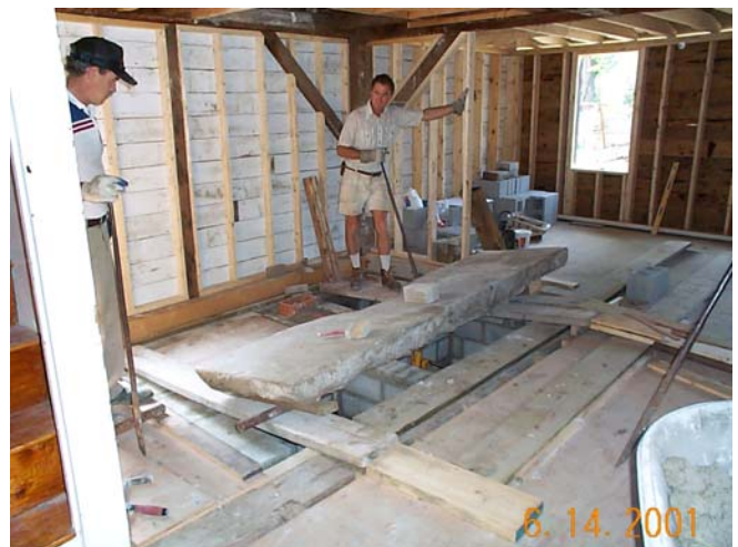
1.28 Ed Gilligan and Graham Pendlebury install the hearth for the missing fireplace in the summer kitchen, June 14, 2001. The hearth was retrieved from the crawl space below.
