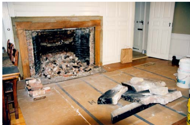
1.24 Dining room fireplace, with Greek Revival mantelpiece and sandstone liner removed, clearly showing paint outline of former Georgian architrave and large brick firebox.
