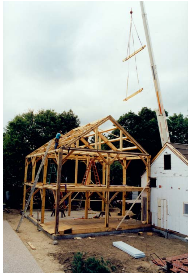
1.36 Barn-raising, September 10, 2001, as seen from the back yard. Will Truax of Center Barnstead, N.H., is coaxing purlins into place. The frame was raised in one day.
